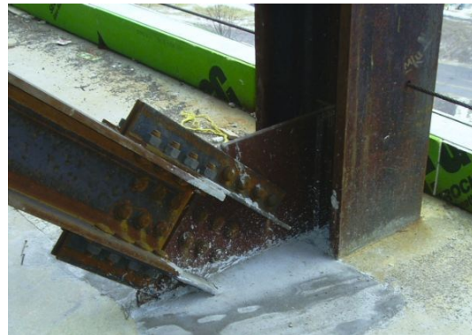
Figure 4 - Diagonal Brace Connection at Column Photo Courtesy of Jim Boje, PE (Wendel)
