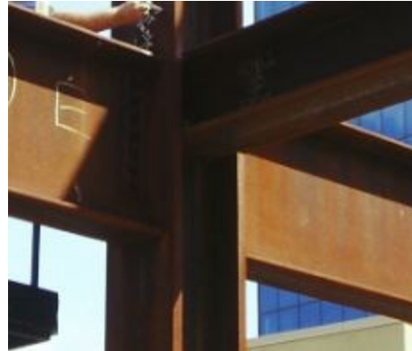
Figure 3 - Typical Moment Connection Photo Courtesy of Jim Boje, PE (Wendel)
